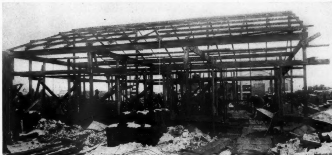
ELECTRIC ARC WELDED STRUCTURAL STEEL FRAME SHOP BUILDING FOR THE C. B. & Q. R. R. AT EOLA, ILL.
